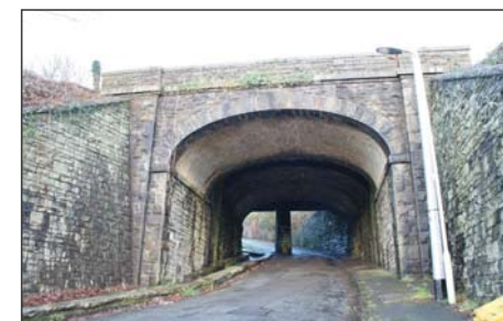
The railway bridge has a distinctive support in the middle of the road!
