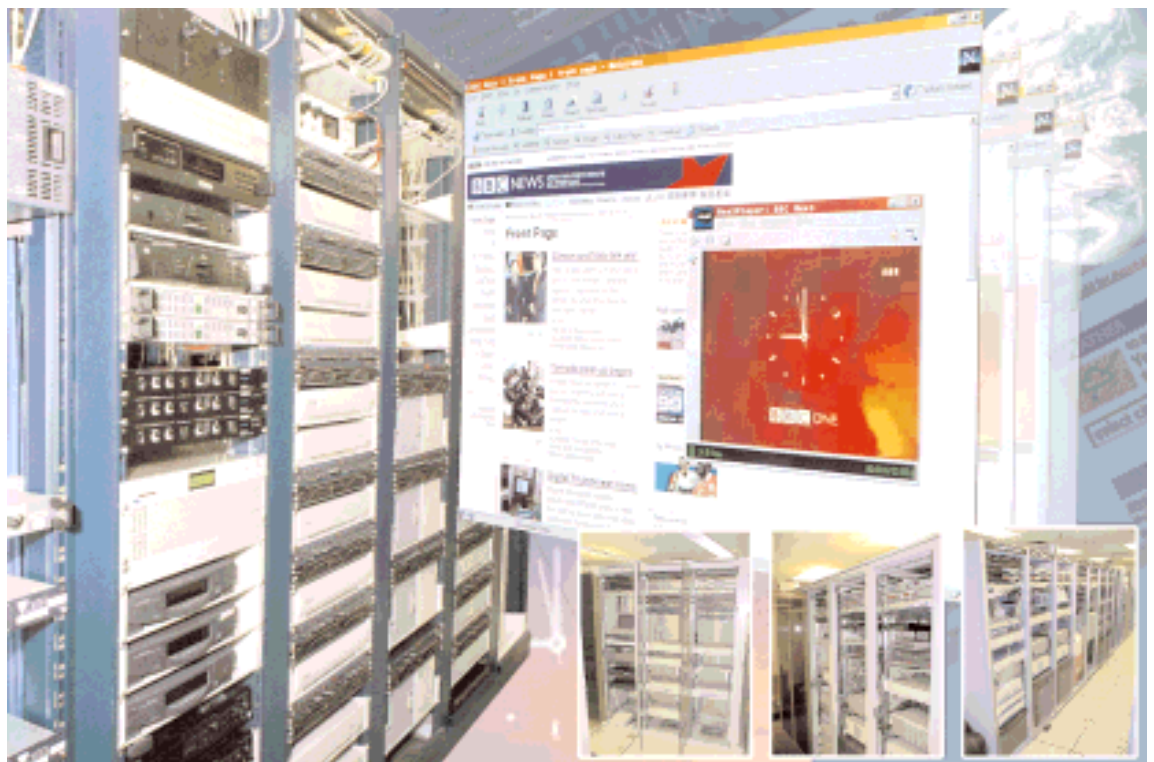
Servers at Kingswood Warren.
